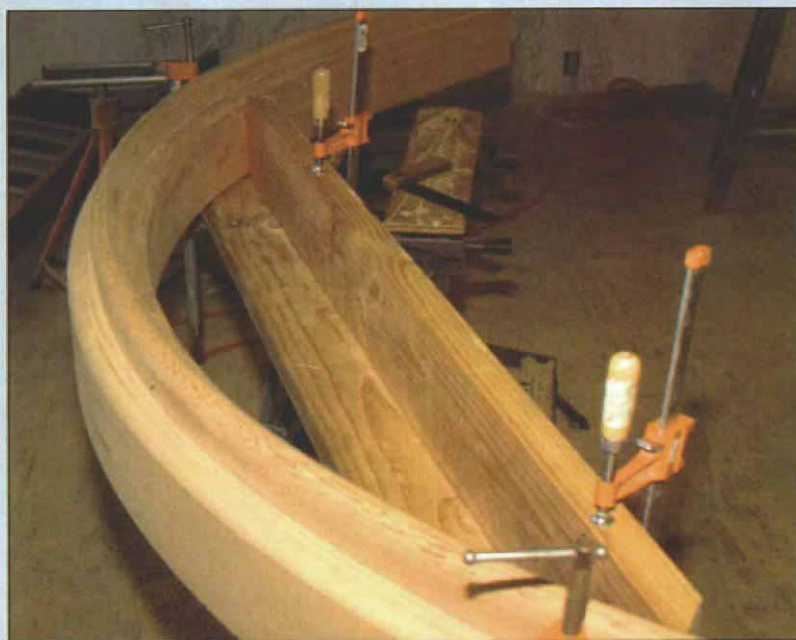
Cutting the curved handrail. A straight jig made of 2x8s enabled the author to find the length and the angles for the curved handrail. After the length and the angles were determined, the handrail was clamped to the jig, and it was used as makeshift miter box.
